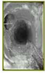
A City sewer main coated with grease
